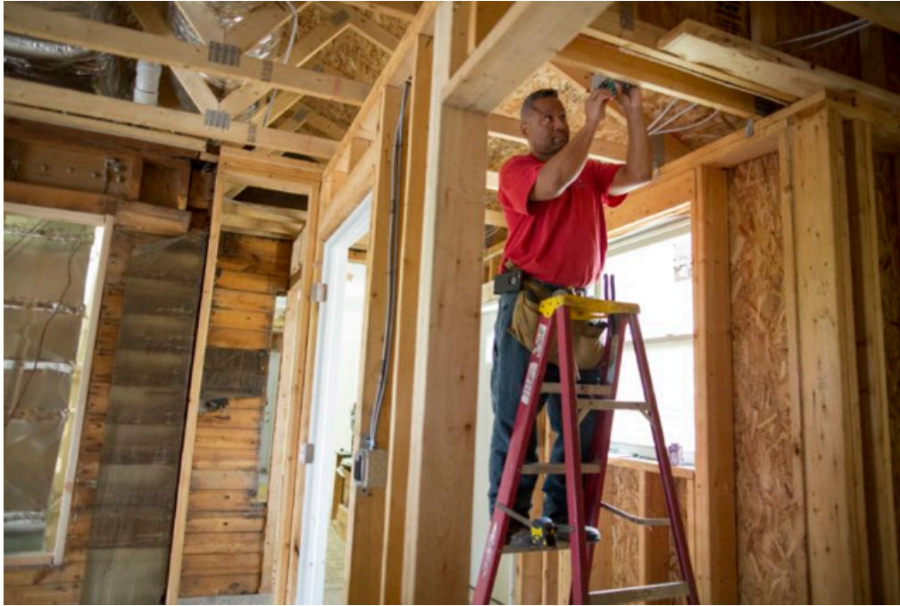
Electrician Michael Watkins wires switches and recessed lights on a new addition at Christ International Community Church. [Adam Cairns/Dispatch]
